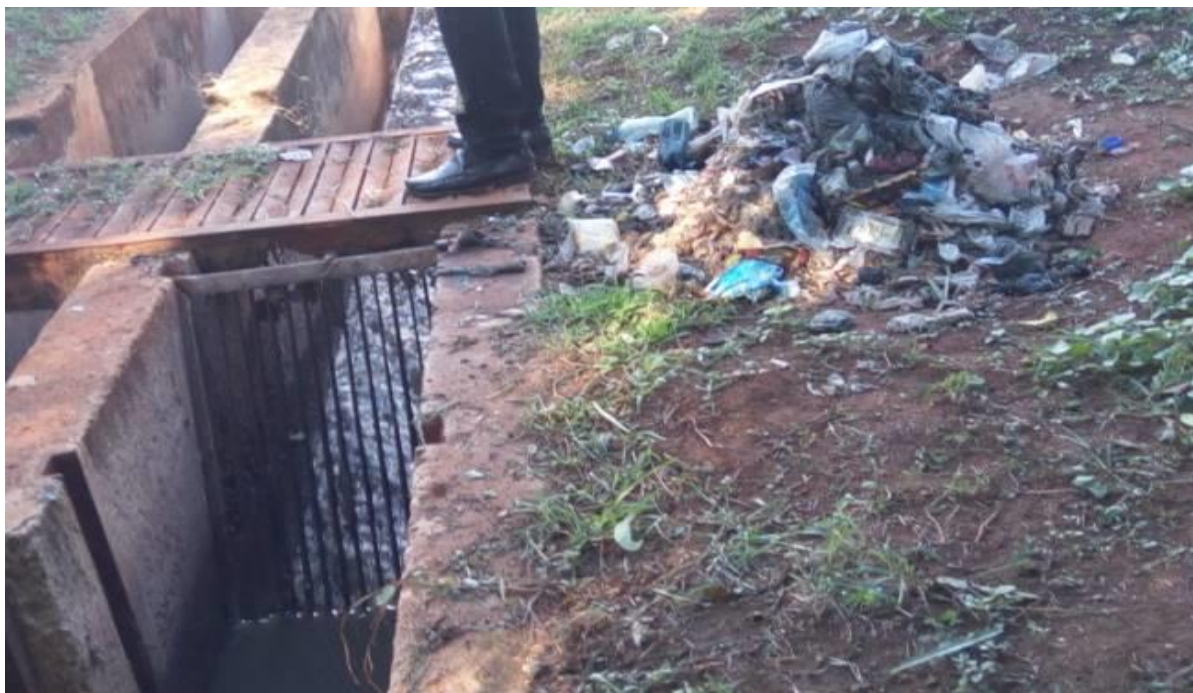
Photo No.5: Screening the influent of solid wastes from entering the waste stabilization ponds
